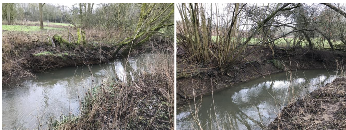
Plate 5: Localised Bank Failure in Process (Left) and Bank Erosion (Right) on the River Ter
